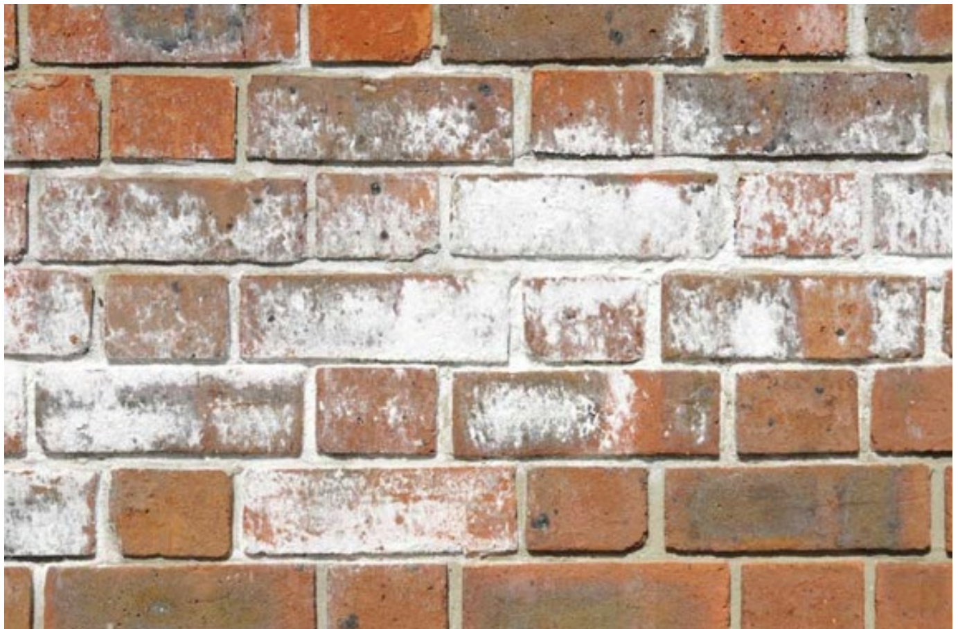
Figure 06 Effects of Efflorescence
