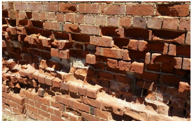
Figure 03 Effects of salt attack on the bricks and mortar
