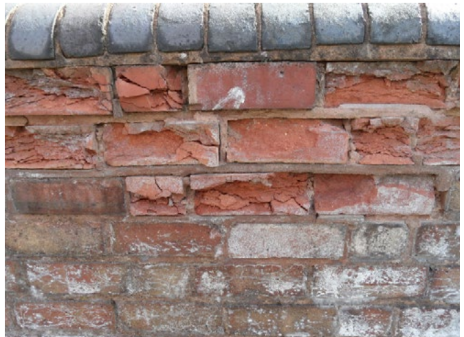
Figure 02 Effects of salt attack on the bricks and mortar
